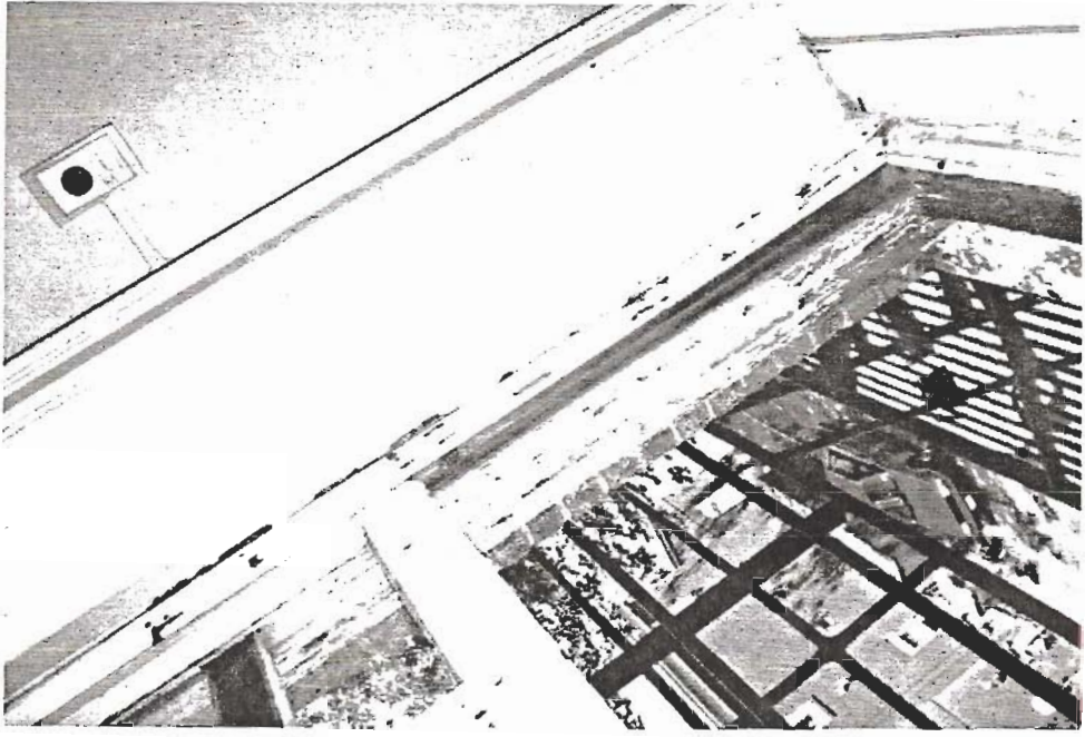
Figure 151 Second Floor: Window Dry Rot.*
