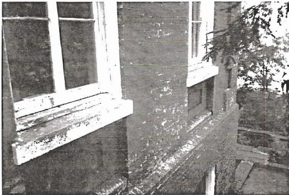
Figure 134 First Floor Window Sill and Recessed Brick Panels, Exterior View, at North Facade.*
