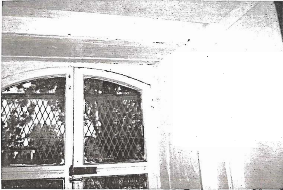
Figure 122 Basement Window Trim Damage.*
