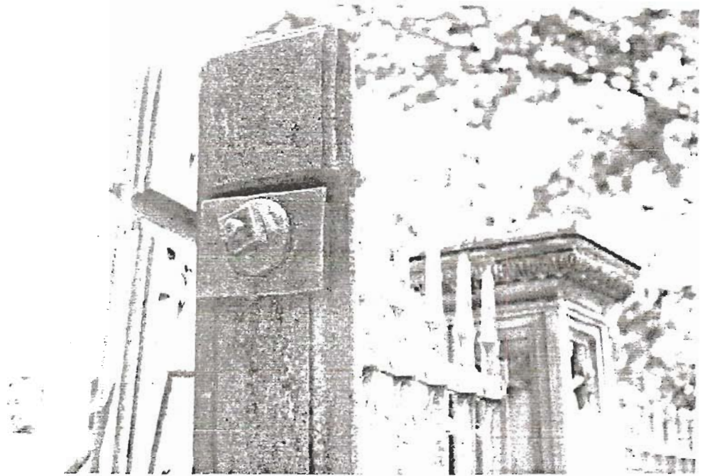
Figure 83 Detail at Capital of Damaged Cast Iron Fence Columns (South Gate).
