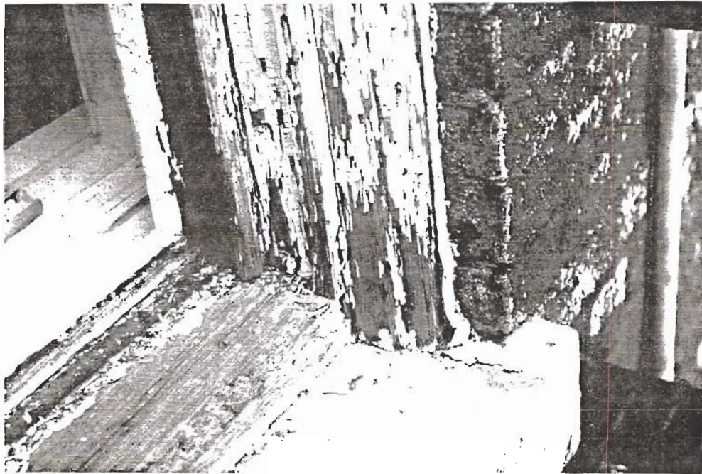
Figure 148 Deteriorated Window Jamb and Sill Detail at East Facade.
