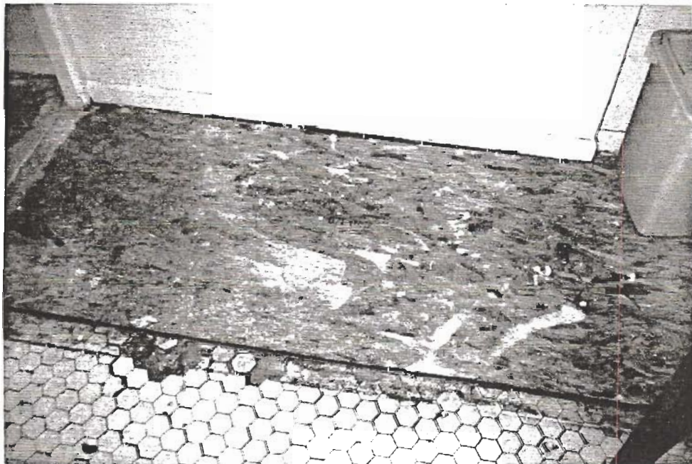
Figure 147 Second Floor: Missing and Damaged Tiles at Women's Bathroom.*
