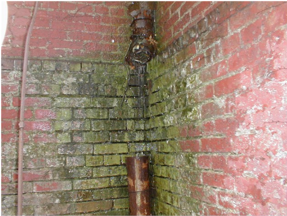
Brick and Mortar Water Damage
